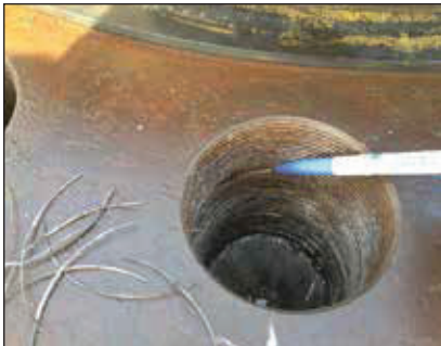
▲ A typical thread before refurbishment
