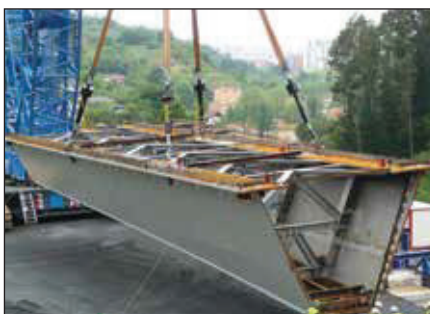
▼ Bridge segments are hoisted from the ground, being positioned with a 4-point SyncHoist system with fully monitored cylinders.
