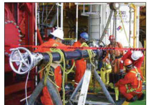
▼ CHT2000 hot tapping offshore application.
